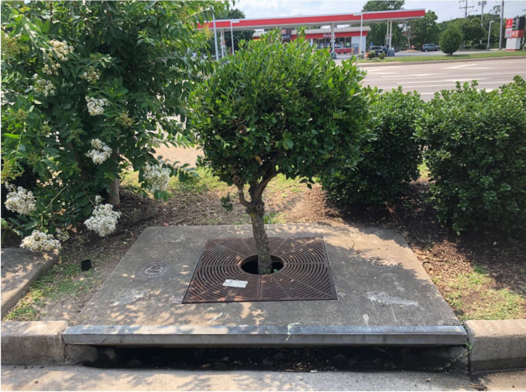
Figure 78. Study site A Filterra system hydraulically tested 2021
