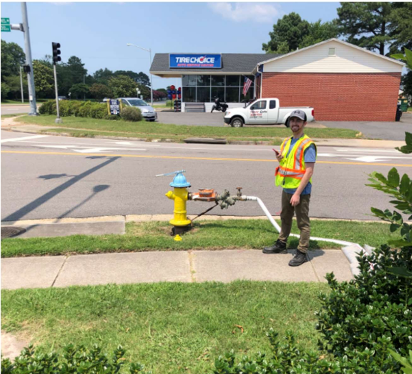
Figure 79. Hydrant and meter set up
