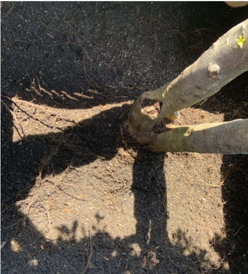
Figure 75. Study site A healthy roots evident post maintenance prior to mulch replacement 2019
