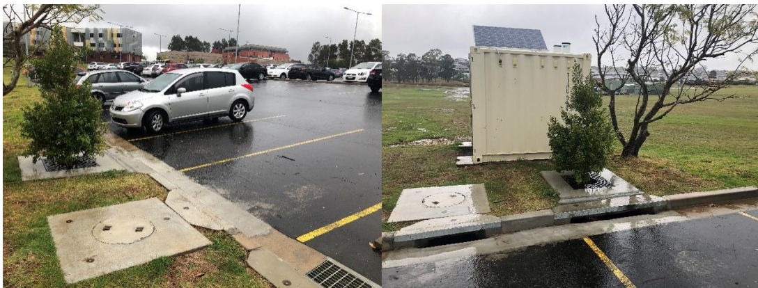
Figure 3: Example photos of the Filterra® biofiltration system and sampling facilities at the site
